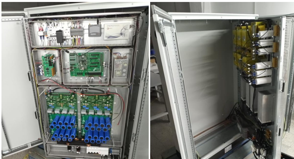
Figure 9: D-STATCOM front view (left) and back side of the mountain plate.
