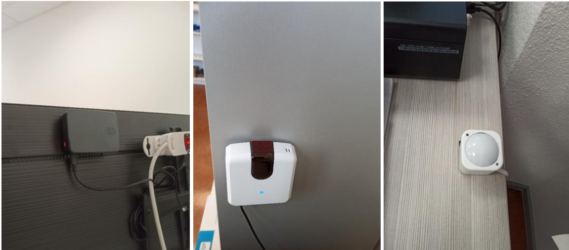
Figure 19. From left to right: IoT Gateway installed in the Municipality building, IR universal control for air condition automatic management, and multisensor installed on desk in office room.
