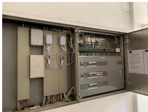
Figure 18. Energy meters connected to the AC units power cables.
